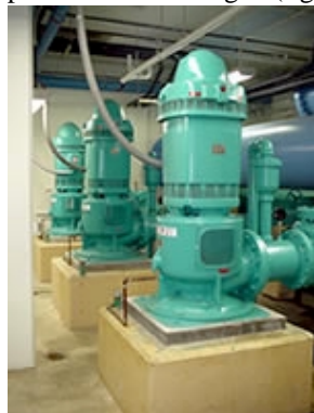
Low service Pumps
