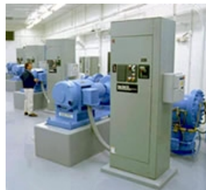
High Service Pumps
