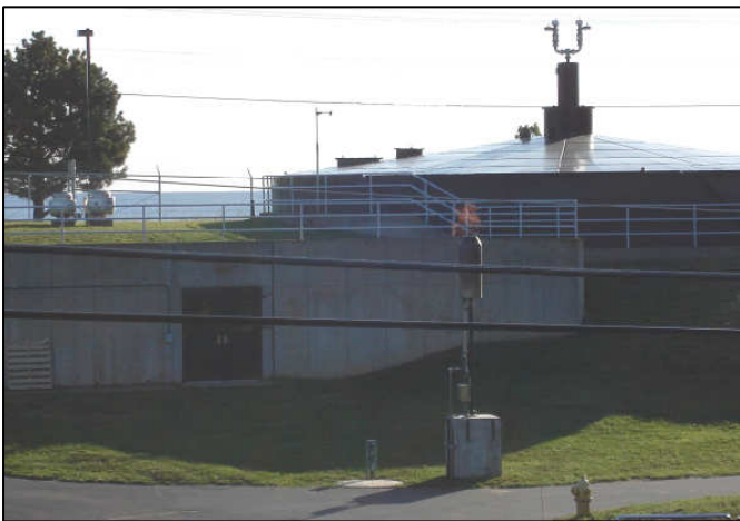
Right: One of three anaerobic digesters at the Marquette facility.
